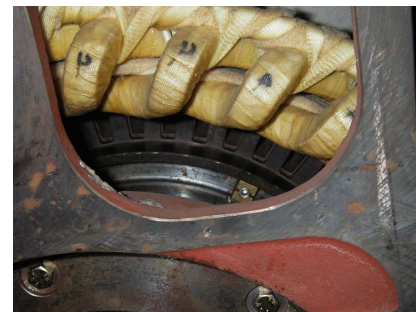
Fig. 3 Induction motor removed cage test
