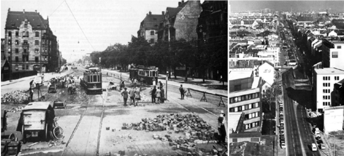
Figure 4 - Fürther Straße before and after construction of the subway (left: Bildarchiv Centrum Industriekultur, right: VAG-Archiv Nürnberg).
